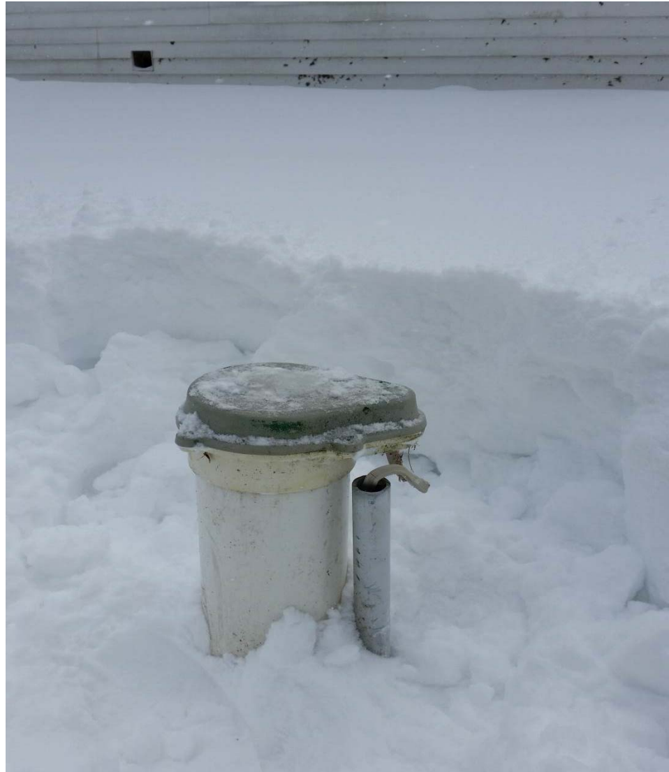
Another damaged well discovered during Point of Sale Inspection. (2-23-15)
