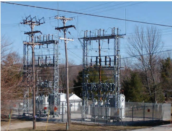
Consumer's Energy substation
