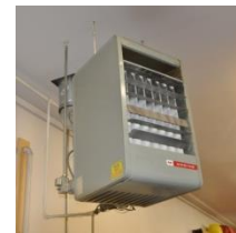
FIGURE 18 - MODINE HEATER IN BAY
