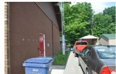
FIGURE 28 - EMPIRE DPW SIDE OF STATION 2
