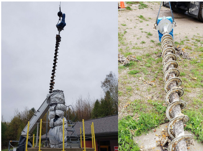
Fine screen auger brush replacement.
