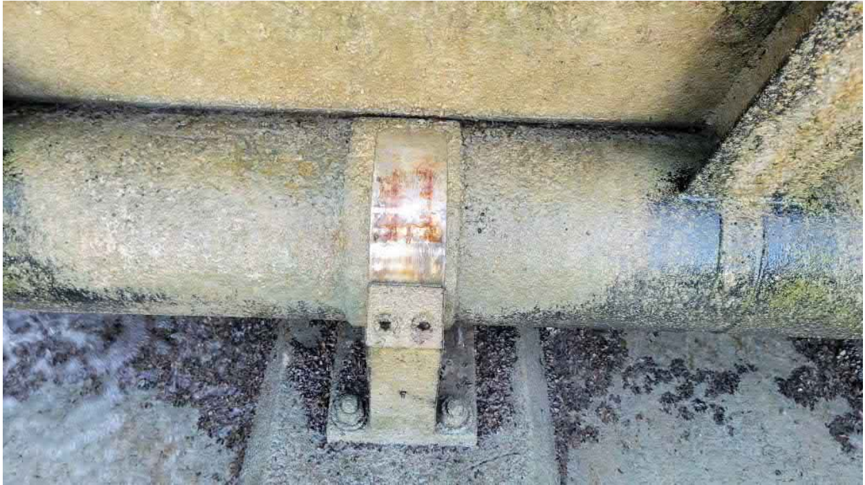
Joint Observation - Corrosion
