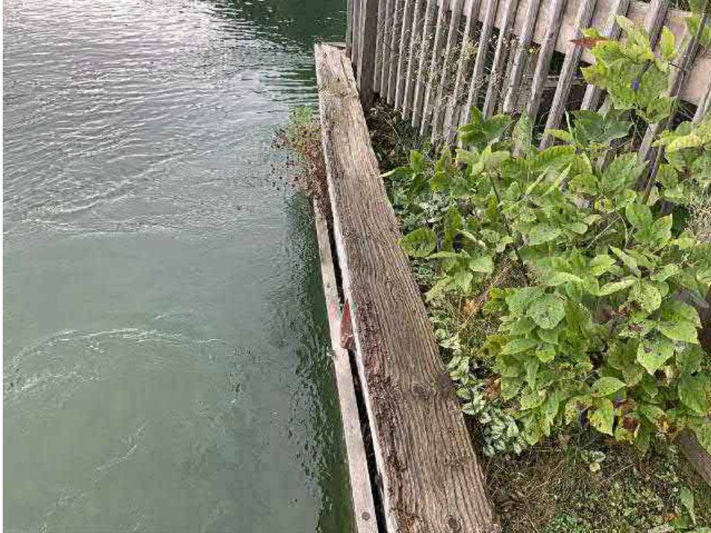
Looking northwest at wooden seawall from northwest (upstream) end of left abutment wall.
