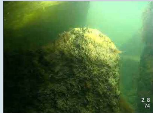
Pier #2 scour wall spall.
