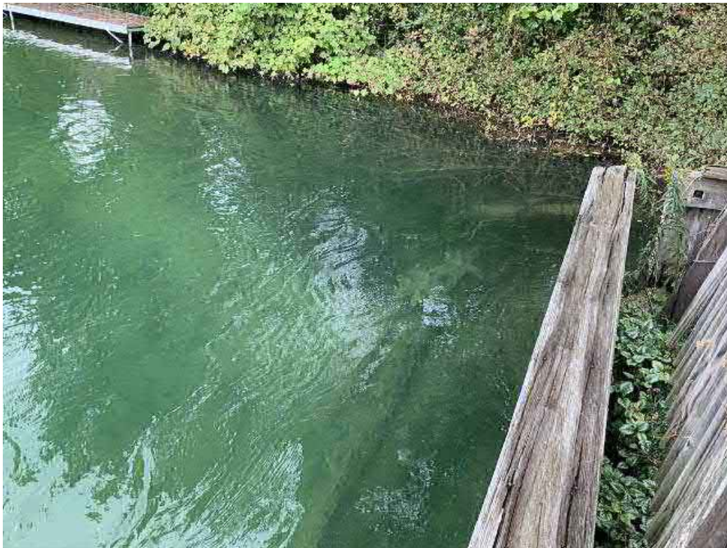
Looking northeast along turned back portion of wooden seawall (left side of channel, upstream of left abutment wall)
