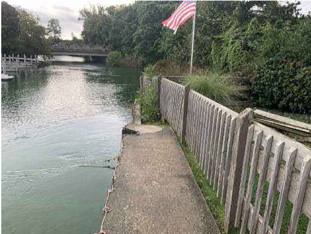
Looking southeast at upper end of left approach abutment wall and wooden seawall.
