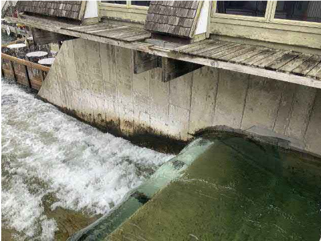
Looking north from walkway at top of actuated weir and right principal spillway abutment wall.
