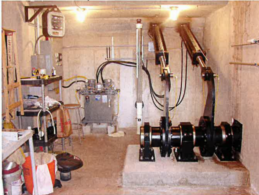
Photo 9. View of automated control panel, hydraulic system, dual rams, gate torque arms and end bearing, and headwater sensor in operations control room.
