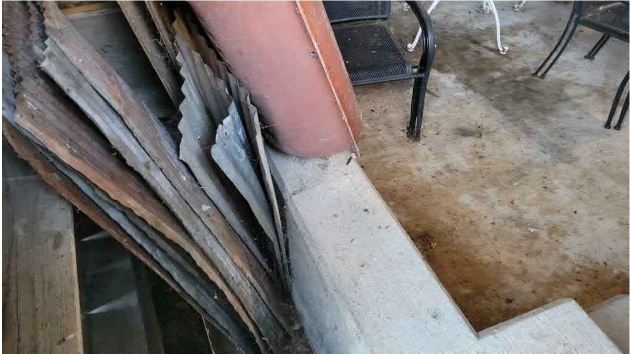
Control Room - Concrete Curb Flood Protection
