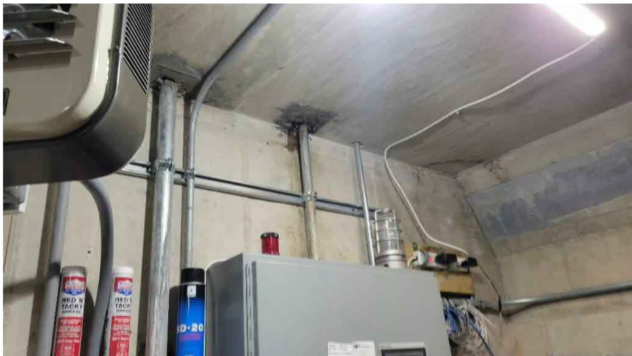
Control Room - Electrical Panel
