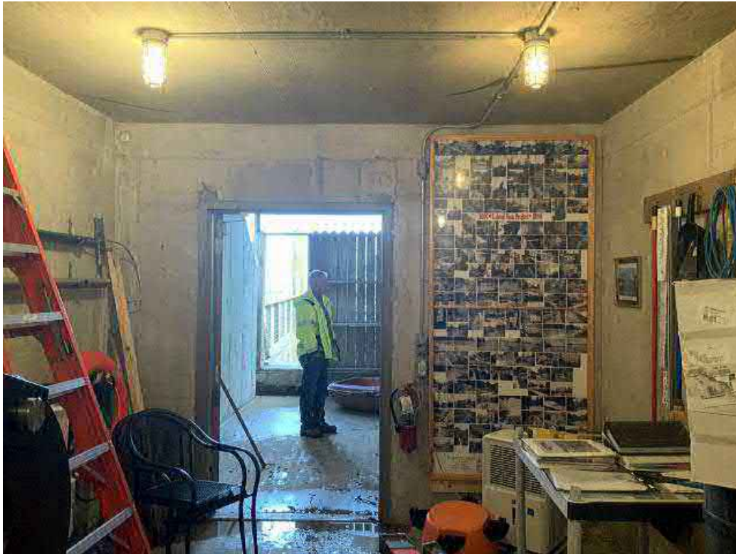
Looking northwest at entrance door and northwest wall of hydraulic / control room.
