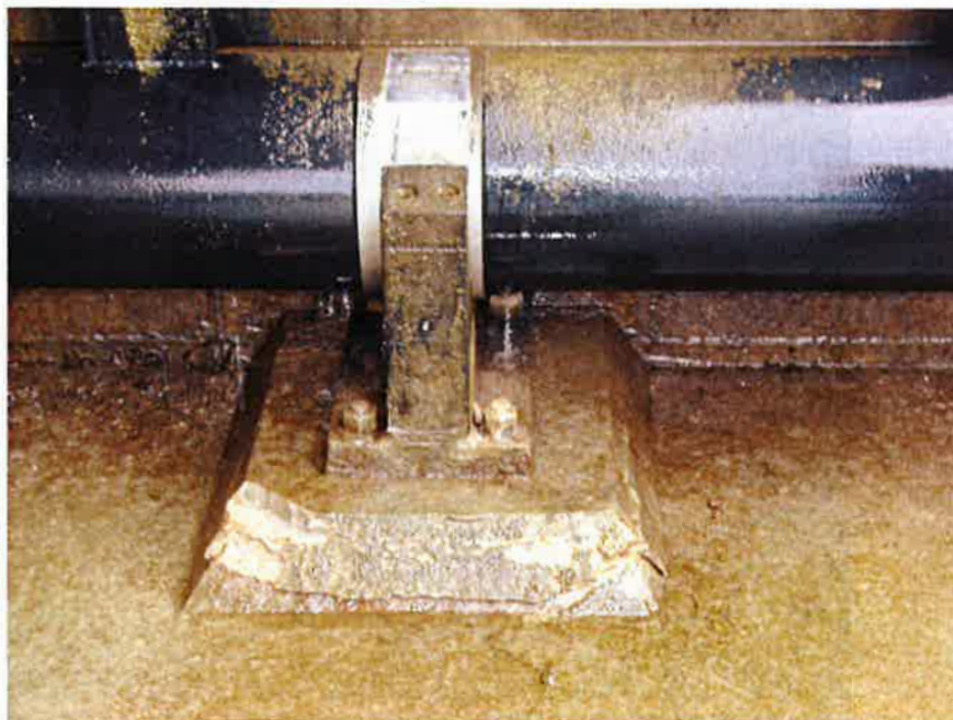
Photo 5. View of spalled grout gate bearing pad.
