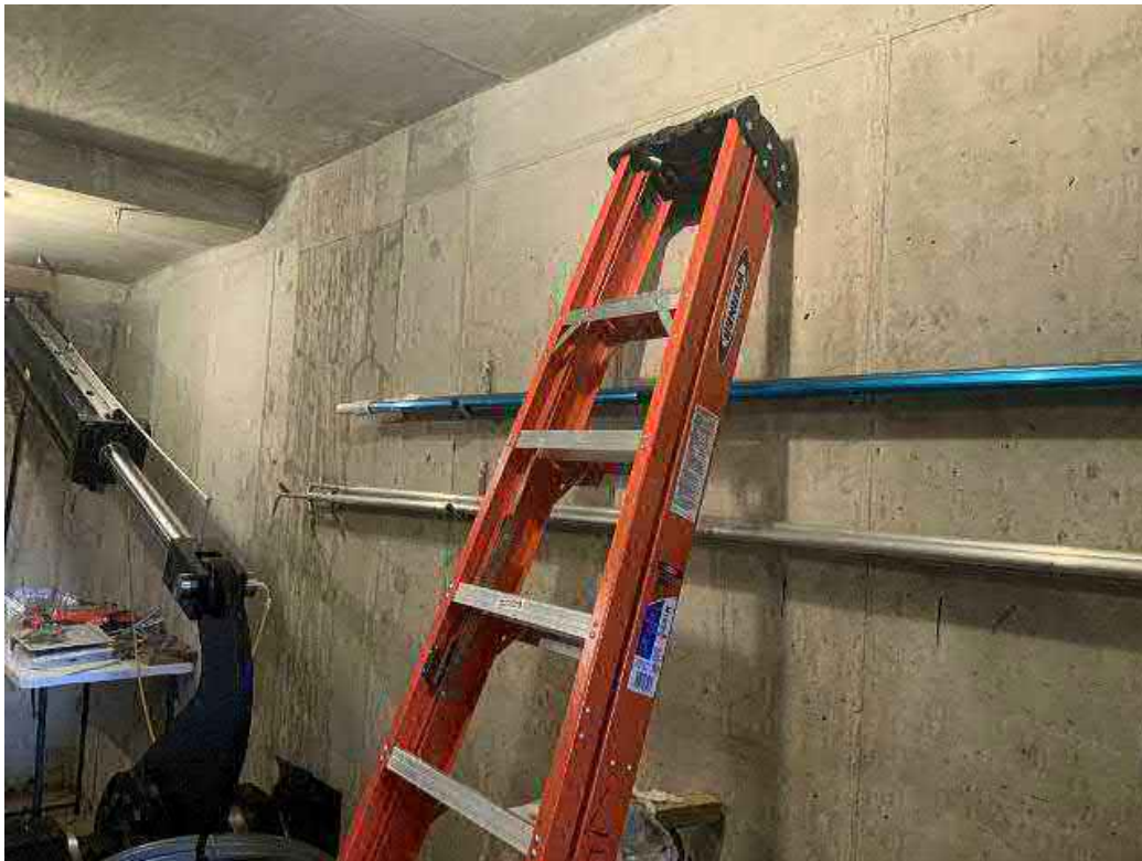
Looking south at south corner within hydraulics / control room.
