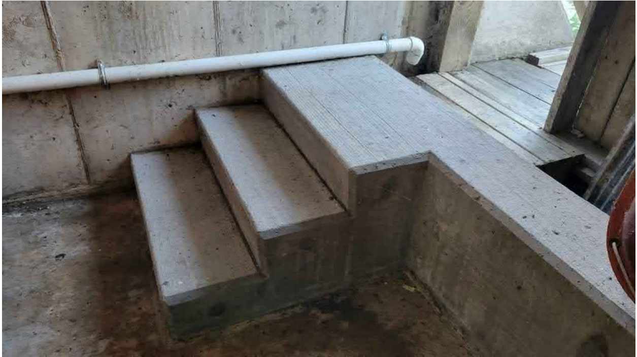
Control Room - Concrete Curb Flood Protection
