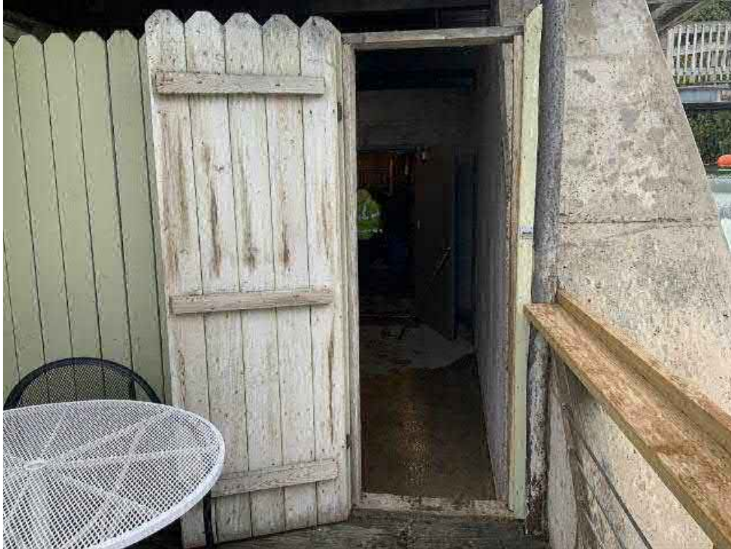
Wooden gate door downstream from just downstream of main door into hydraulics / control room (former Bay #4).
