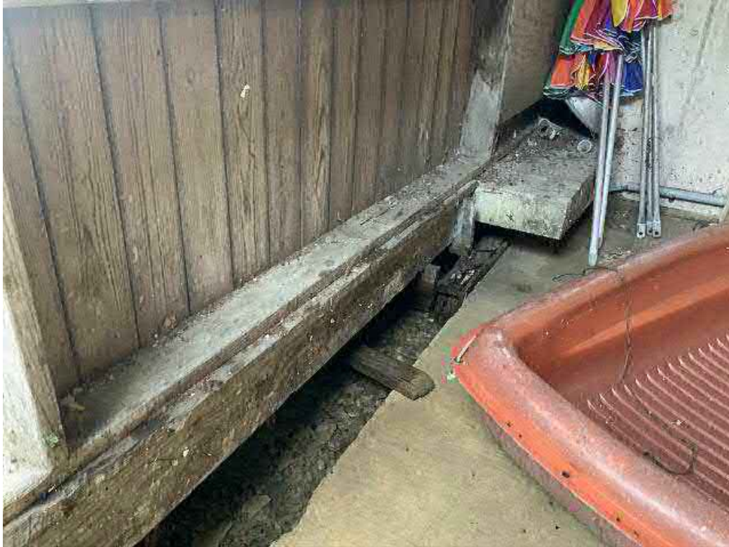
Looking northeast along former downstream end of Bay #4 spillway, downstream of hydraulics / control room.
