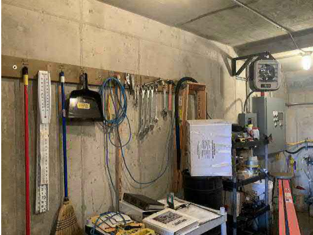
Looking east at corner of hydraulics / control room.
