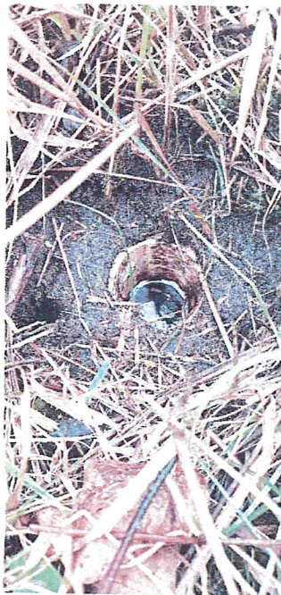
Broken well casing pipe.
