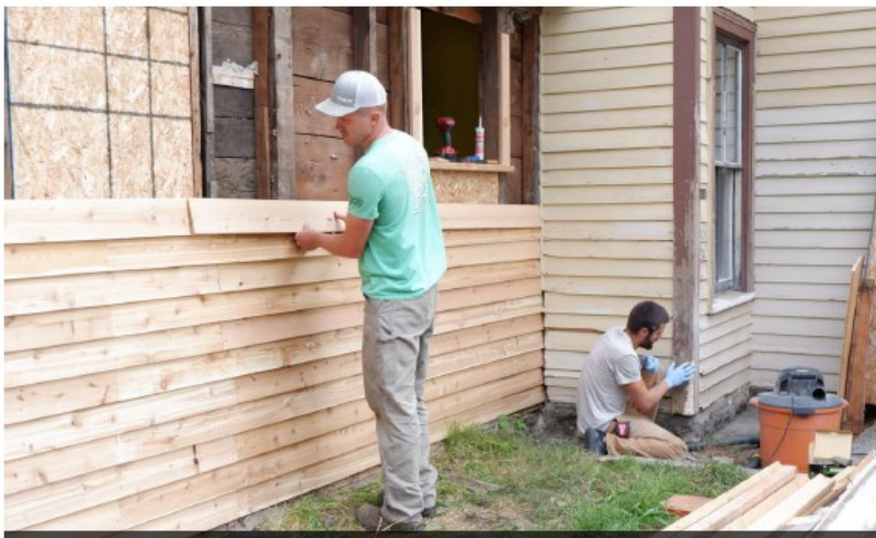
Still to do: Siding repair and lots of finishing touches inside. On the list: Insulate the walls, replace windows upstairs due to safety concerns, plaster, drywall, trim, floor refinishing, and a new kitchen.
