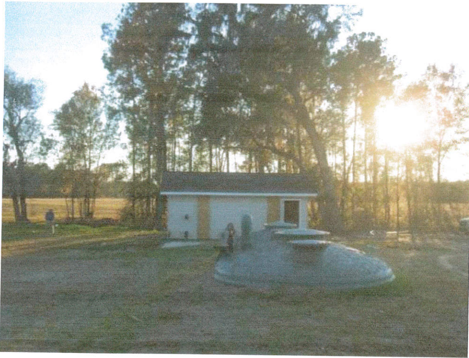
Typical clarifiers and control building
