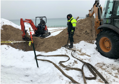
Jan 23, 2020 Drain Plugged, Channel Closed Two Workers, Firehose, Equipment Required
